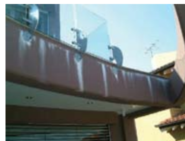
Photo 6. Where the gradient in the substrate leads to a free edge, efflorescence will form on the riser. To avoid this problem, seal a water-stop angle to the floor at the edge or one tile in from the edge, and grade the substrate behind the angle to a drain.
