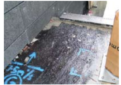
Photo 7. A gutter down the left edge of the stairs, which contains drainage cell material under the stone, will ensure that water from the landing takes that pathway and does not emerge through the stair risers.
