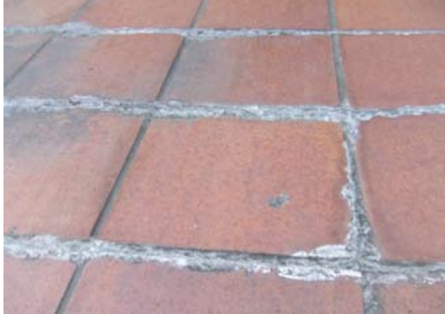
Photo 2. Efflorescence forming where moisture below the impervious tiles rises through cracks in the grout.
