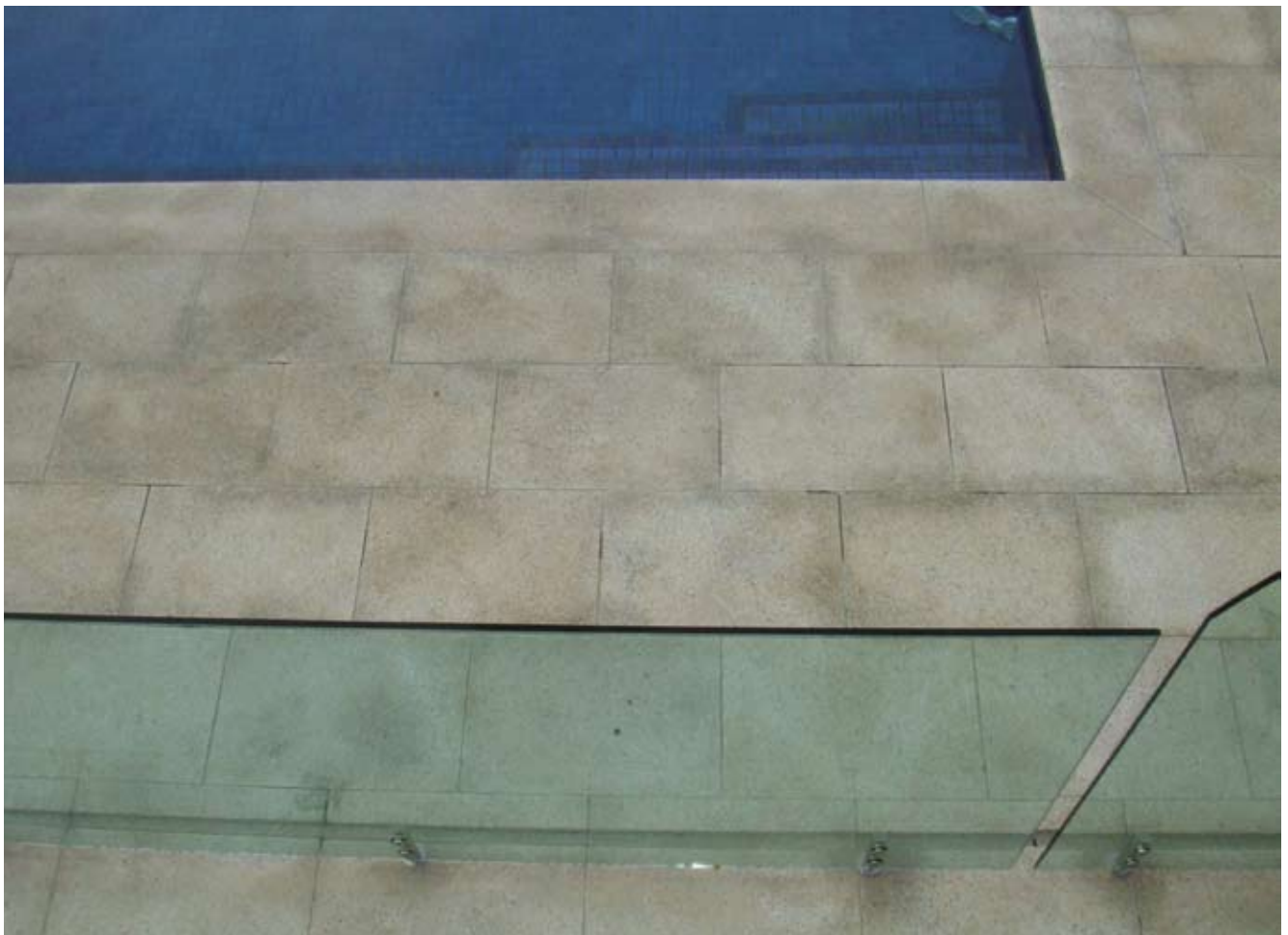
Photo 9. Efflorescence has formed inside this granitic stone and it is now irremovable. Pre-sealing the back of the stone with a specialist solution could have avoided this problem.
