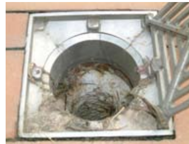
Photo 5. When the drain is open at the neck, and there is a gradient in the substrate to the drain, the efflorescence forms down the drain pipe and not on the tiles.
